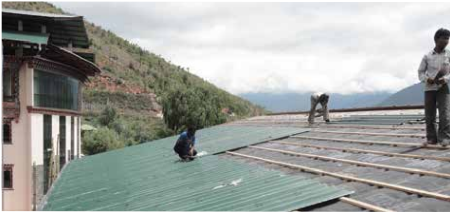
Ventilated roof construction with waterproof underlayer preventing moisture to get in contact with the timber trusses below. A roof is a potential surface to integrate solar elements to produce hot water and /or electricity
