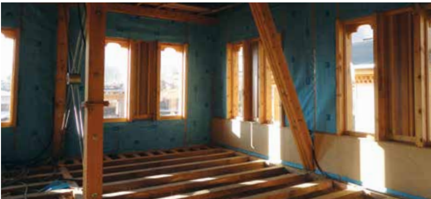
Timber construction with thermal insulation and vapor layer on the room side
