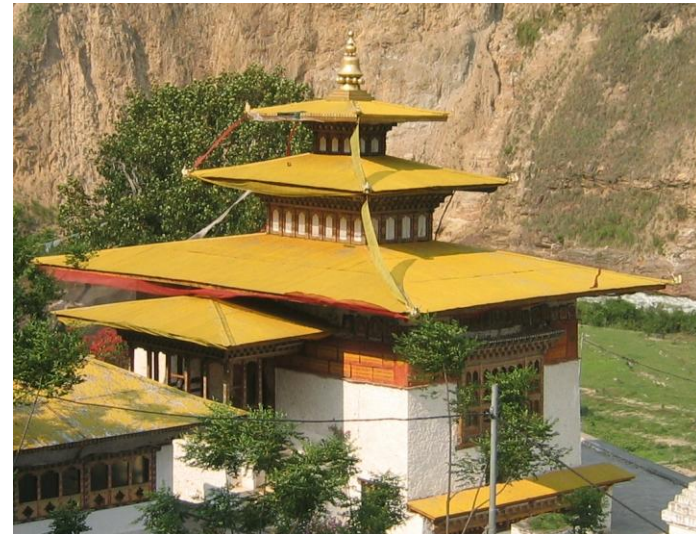
Jabzhi Roof over Goma Kora Lhakhang in Tashi Yangtse (Picture: Dorji Yangki)
